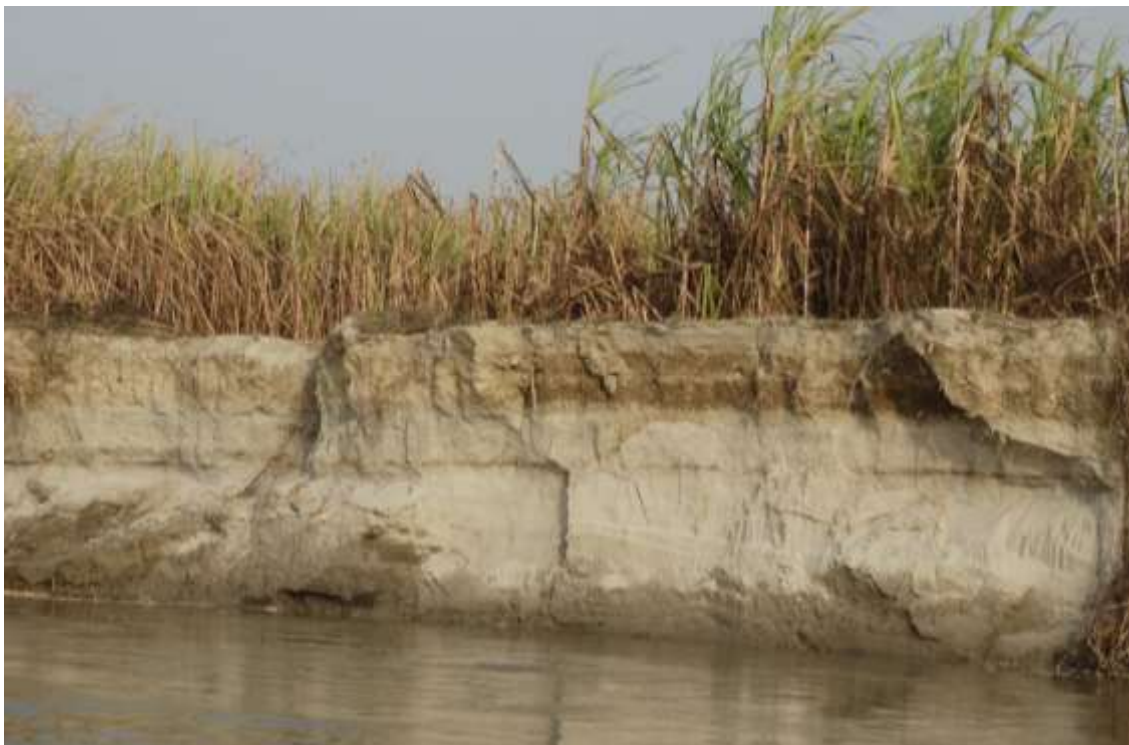
Image 33 : Lateral Bank Erosion Near Nizampur
